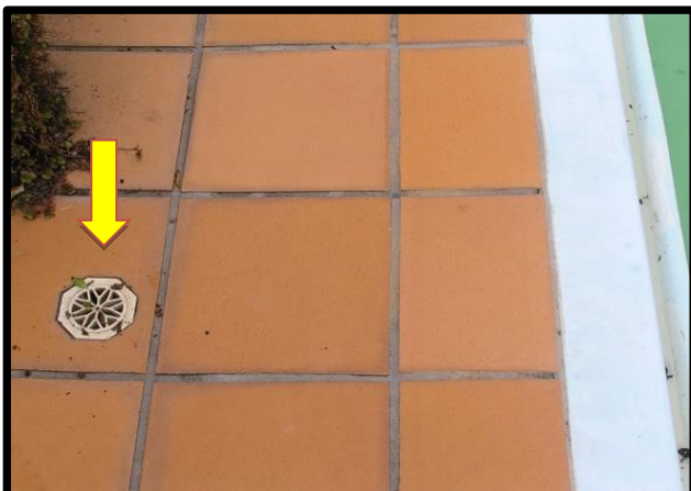
Fig2: A grating covering a tube near the pool to check the water table – level. (See arrow) You can insert a hose here and pump out if too high. Will take time so do a few days before you want to empty the pool.
