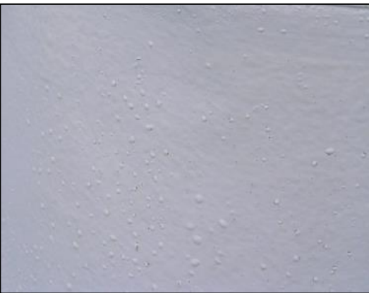
Figure 5 Painted wall showing hydrostatic blisters
