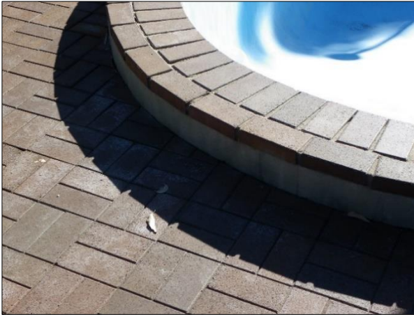
Figure 1 Dark pavers and coping with efflorescence present, with drainage. Resulted in blisters on pool walls
