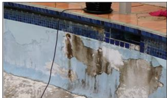
Figure 4 Effects of poor drainage around pool and causing in part delamination of render.
